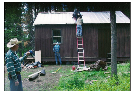
Repairing the metal roof. Don Barth is on the roof, Don Dodge on the ladder, Richard Tamcke painting, Paul Evenson working on the deck and Mack Long in the foreground.
