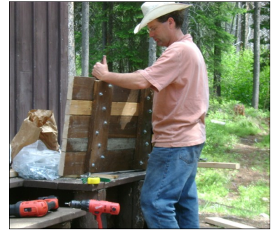
Above, Scott Tuxbury making new shutters for the old cabin windows and door.
